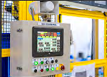
Process Automation System
